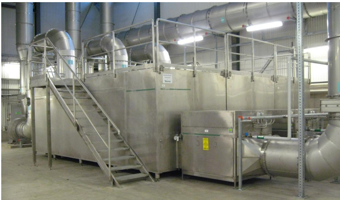
Figure 7. Combined photo-oxidation and carbon filters
