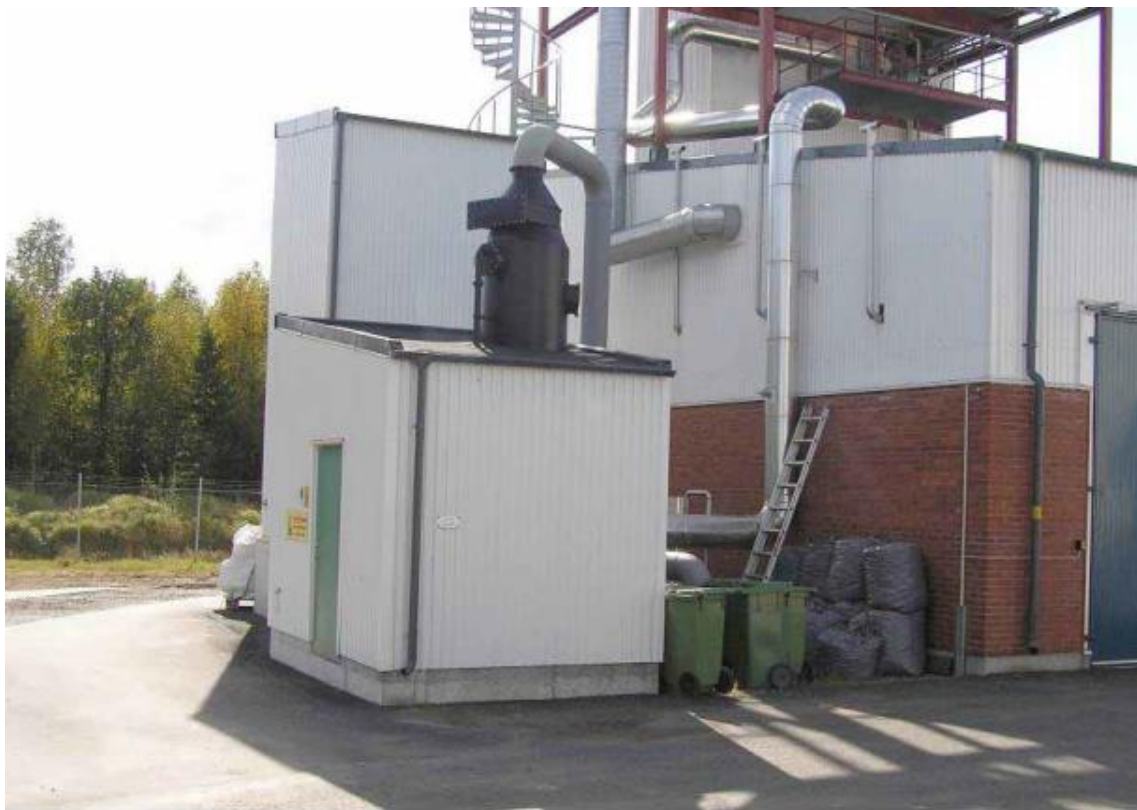
Figure 3. Chemical scrubber installed at the upgrading facility at an anaerobic digestion plant in Sweden (Photo: Swedish Waste Mgmt Assoc).
