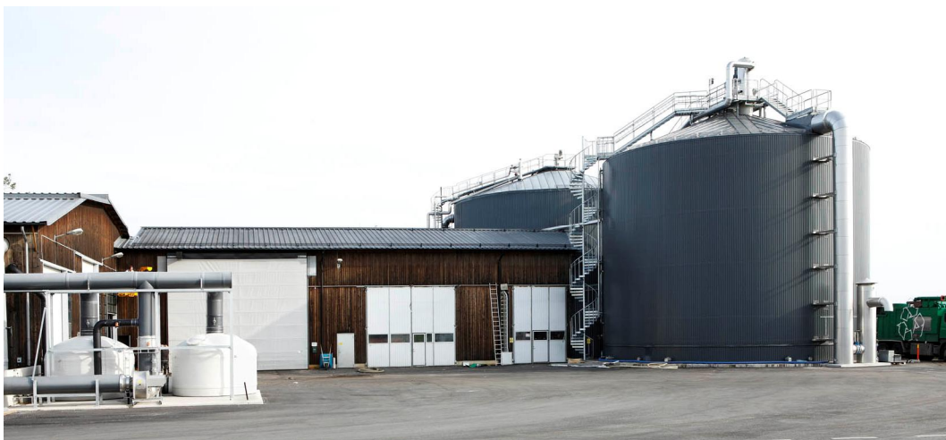
Figure 6. Carbon filters (to the left in the picture) at the Uppsala anaerobic digestion plant for food waste from households.
