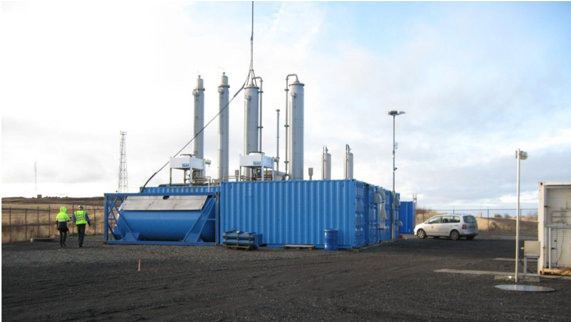
Figure 12 Gas upgrading plant for landfill gas
