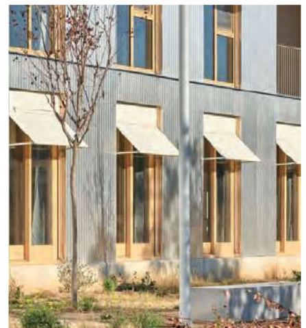
Plinth with different colour foot, relating to the colours of the rest of the building
