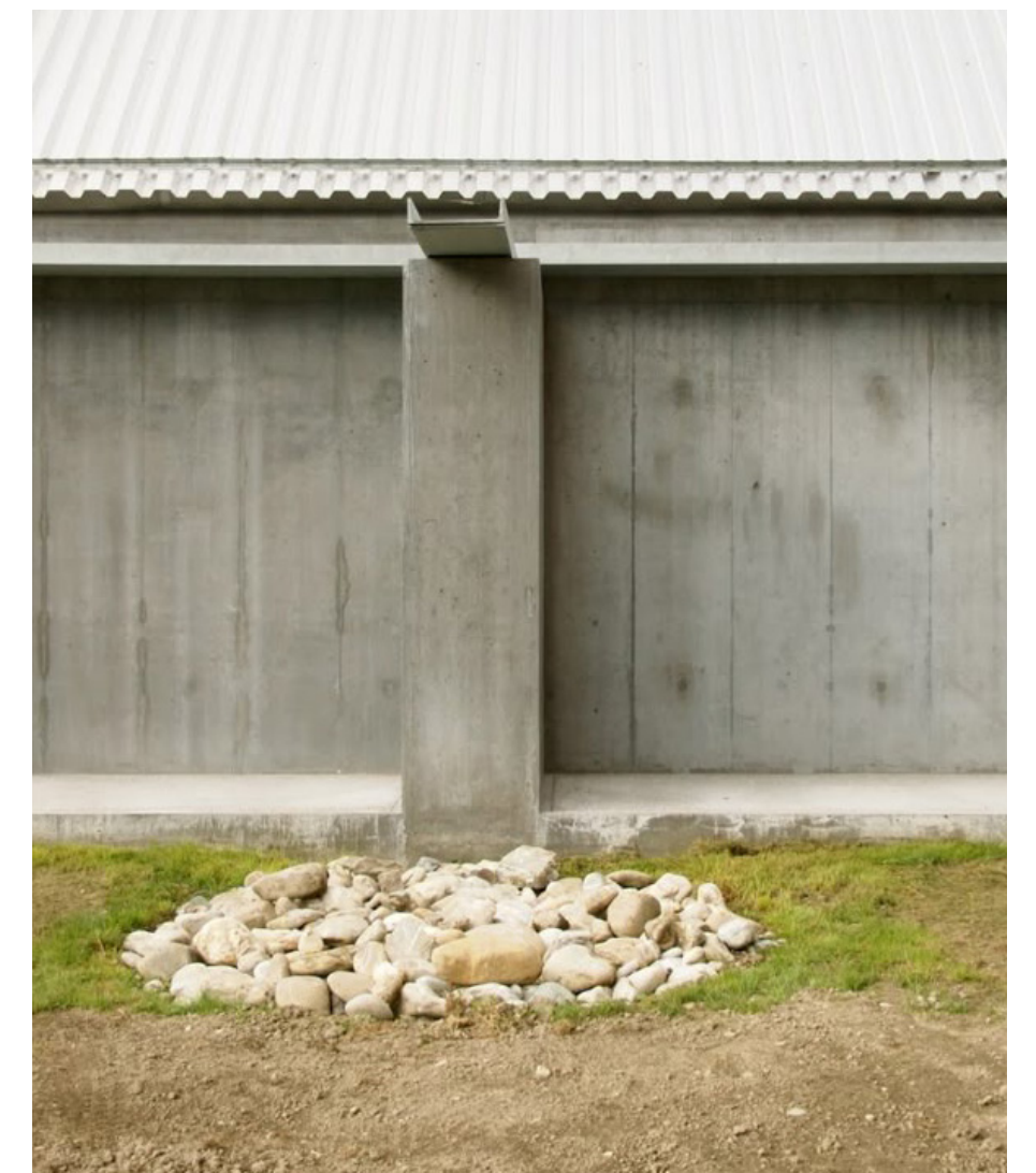
Architectural overflow to podium deck
